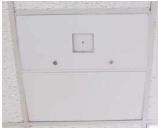
Rc142 Drop Ceiling Repeaters
